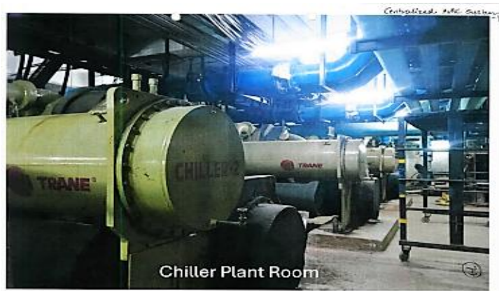
CHILLER PLANT ROOM
