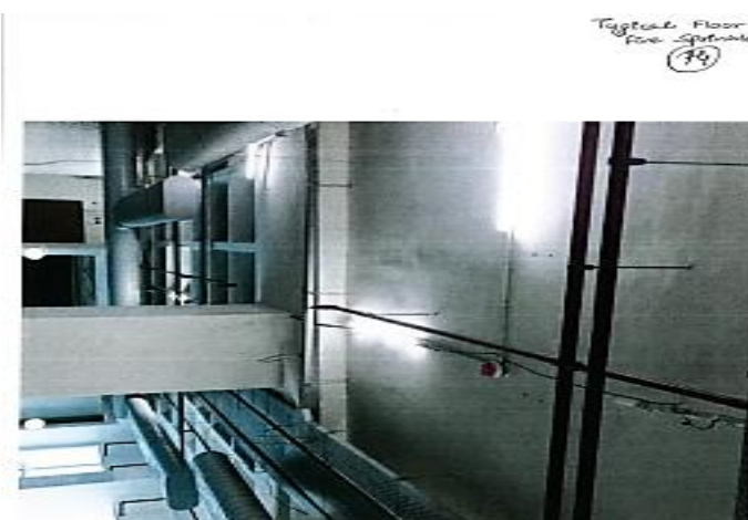
FLOOR FIRE SPRINKLER
