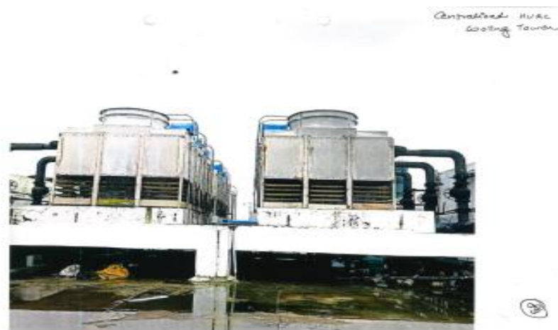
CENTRALISED HVAC COOLING TOWER
