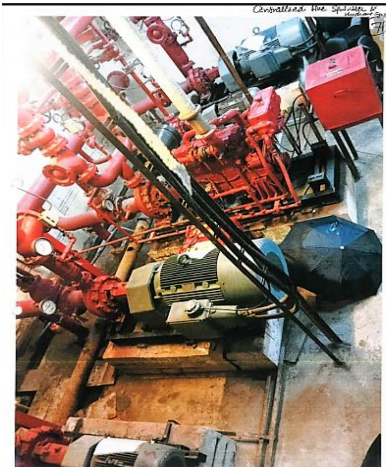
CENTRALISED HVAC SPRINKLER
